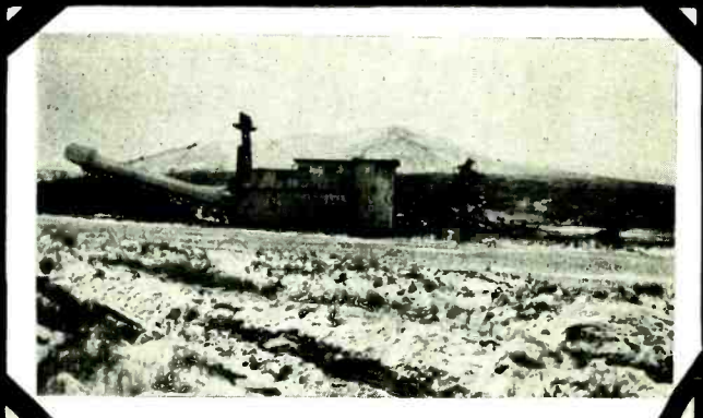
(Above) A half-million dollar dredge at Goodnews Bay. The machine is over 60 feet high, operates day and night, can dig 50 feet into the earth, requires a 25-man crew to run it.
